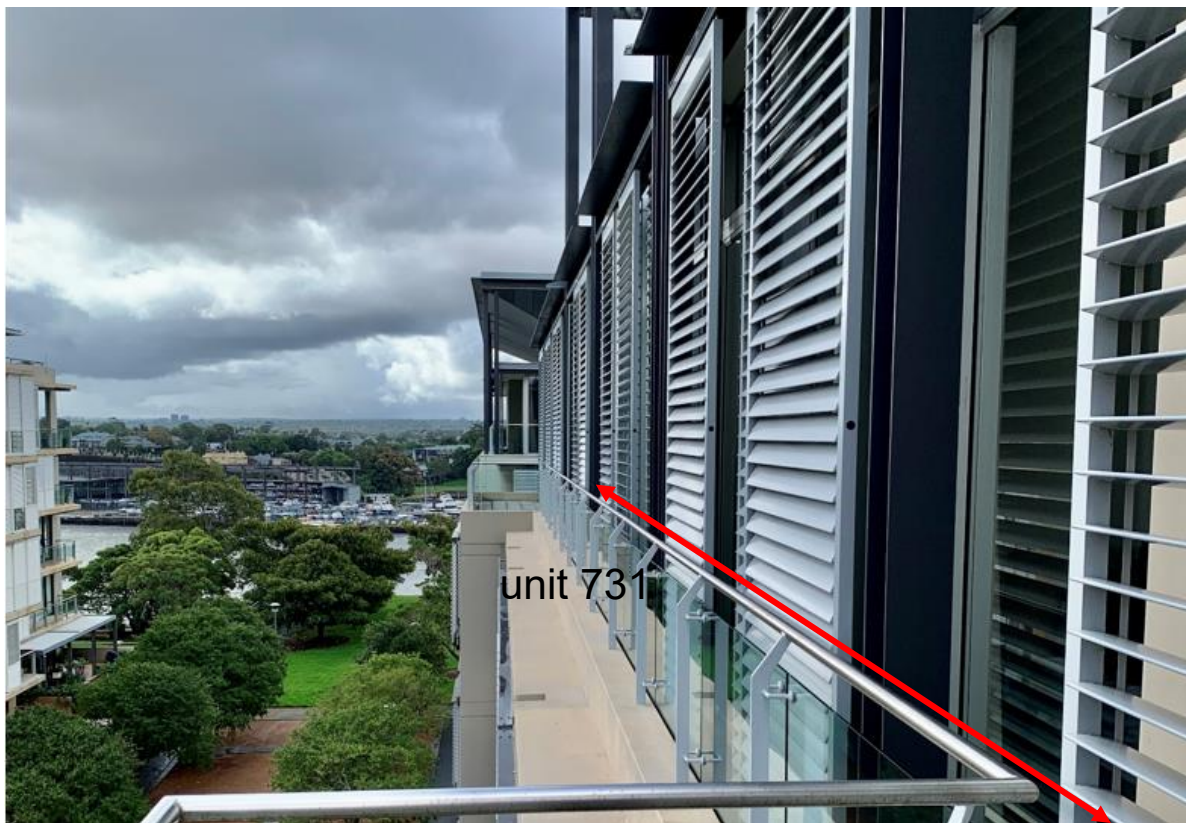
Figure 9: West elevation of Unit 731, including the existing shade devices, as viewed from western end of the private terrace
